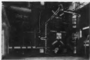
B&W waste heat boiler conditions flue gas for air heater and produces enough steam for plant base load requirements.
